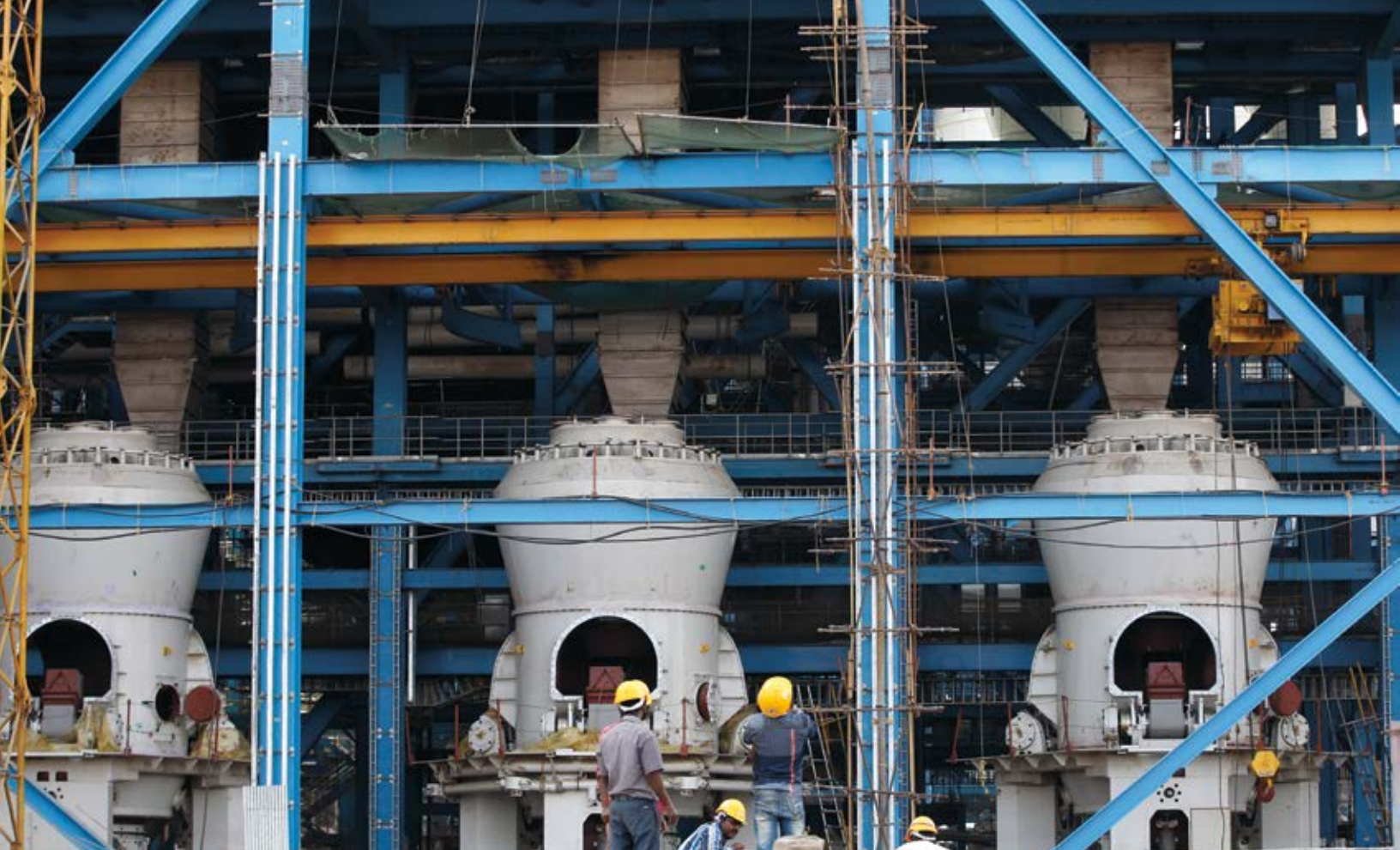
Boilers are seen being installed at the under-construction coal-fired power plant, partially financed by the Japan Bank for International Cooperation, in Kudgi, India. ©AP Photo/Rahi
