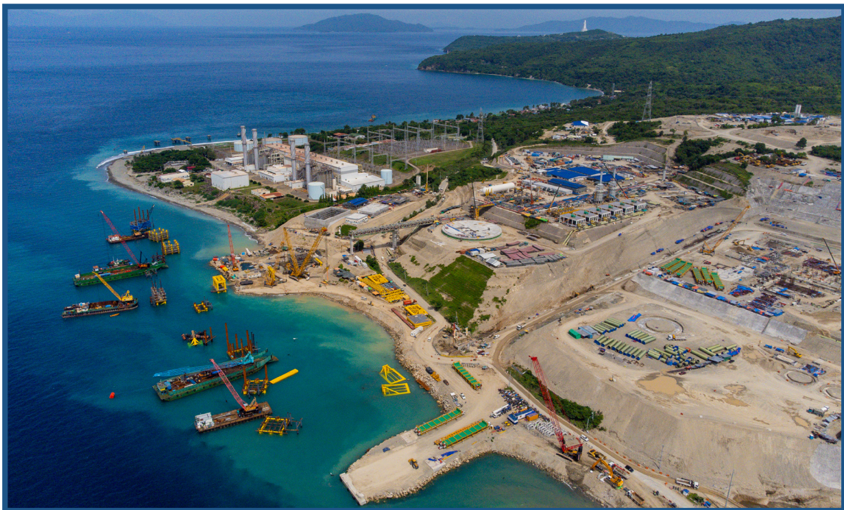
Construction of a new gas-fired power plant and LNG import terminal is seen in the province of Batangas, south of Manila, Philippines. Source: Basilio Sepe
