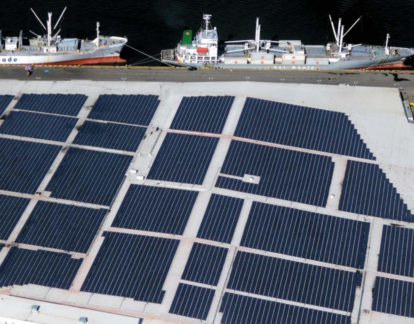
Solar voltaic panels. ©Associated Press
