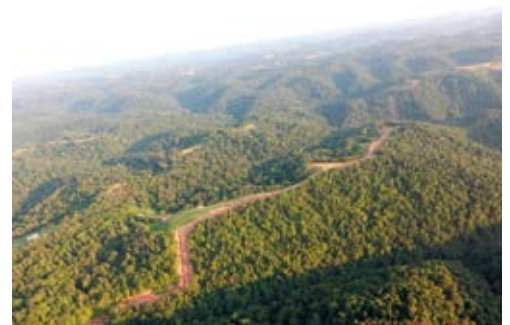
Cross-country pipe being installed. ©Ed Wade, Wetzel County Action Group, FracTracker Alliance
