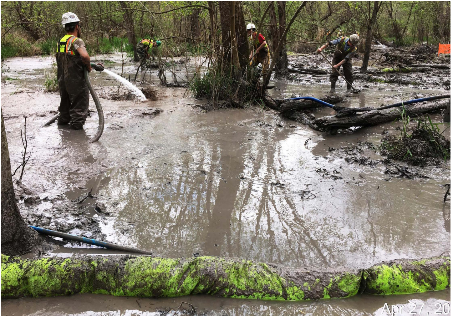
Crews in Ohio clean up a spill of millions of gallons of drilling waste caused by construction of the Rover Pipeline in April 2017. ©Ohio Environmental Protection Agency.
