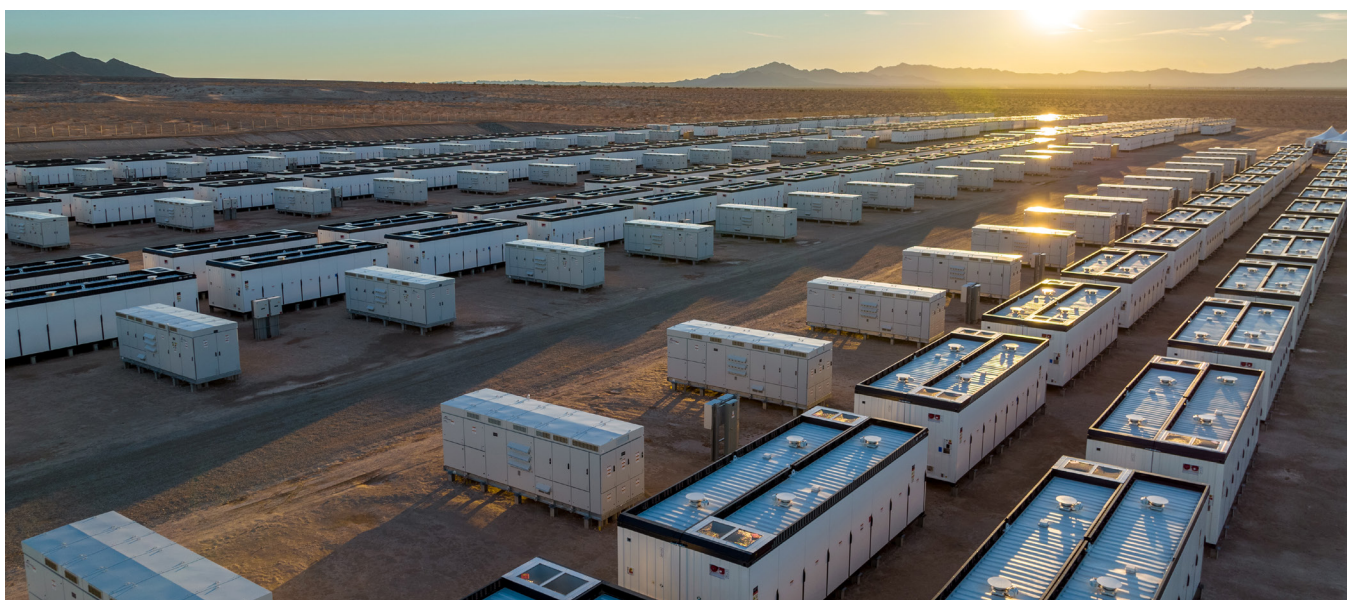
The Crimson Energy Storage Project, a 350 MW battery storage system for Crimson Solar in eastern Riverside County, California. Source: Bureau of Land Management, Flickr.
